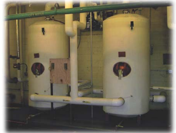
Two Raypak 534 gallon storage tanks are maintained at various temperatures depending on demand history.
