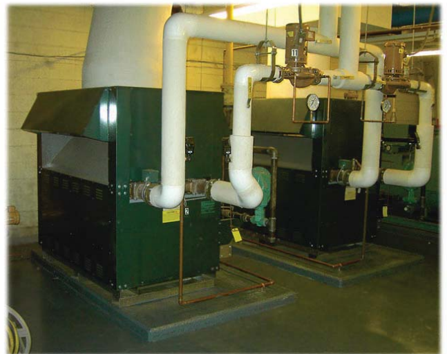
Two Raypak WH-2500 water heaters provide hot water to the guests rooms and kitchen area in the 376-room hotel.
